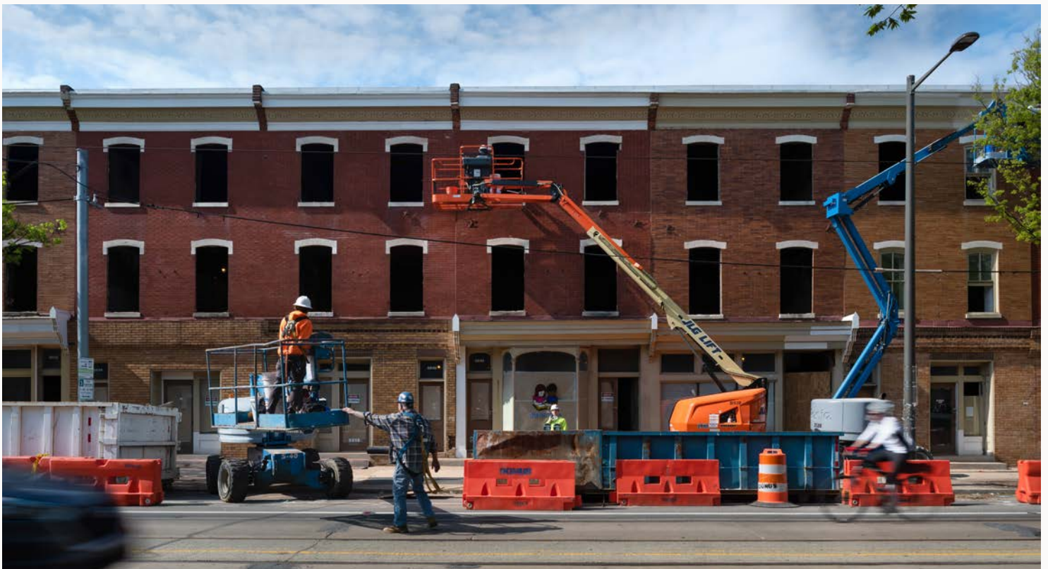
A construction team renovates historic rowhomes in Powelton Village in West Philadelphia into student housing near Drexel University and the University of Pennsylvania. [Photo by Kat Kendon, April 2019]
