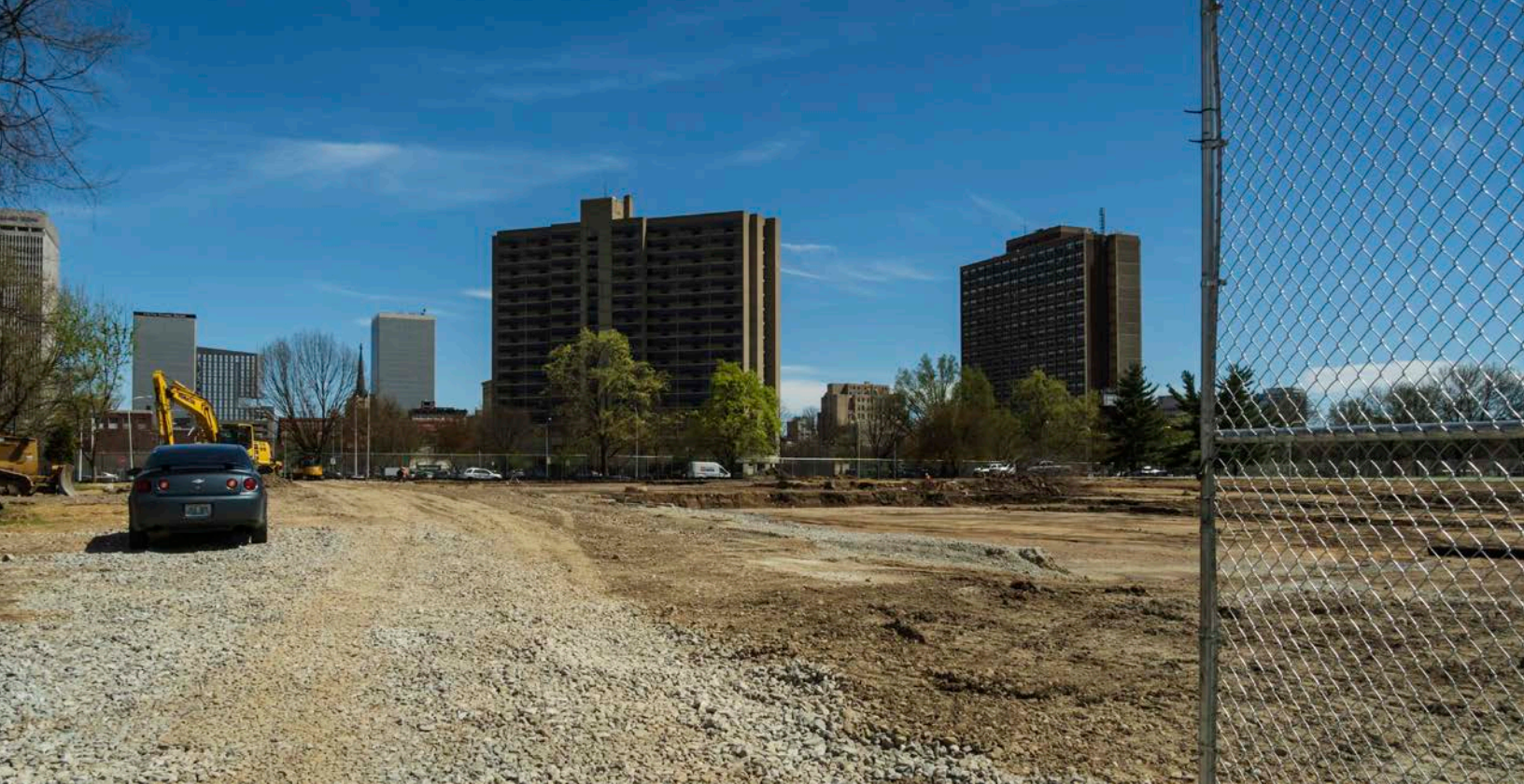
The Louisville Metro Housing Authority received Choice Neighborhood Initiative Implementation grant funding from HUD to demolish the distressed Beecher Terrace housing complex, built in 1939, and redevelop it as mixed-income housing. [Photo by Andy Snow, April 2019]
